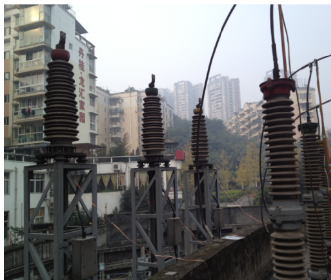
Figure 11: Shuhui Line cable termination, the 122 equipment interval of Huidong Substation
