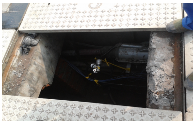
Figure 14: China Mobile was distal, the metallic protective layers were all short circuited and suspended
