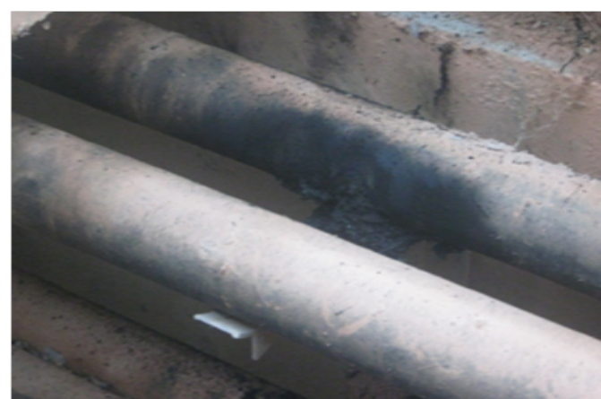
Figure 18: Fault points of single core cable outer sheath layer discolored by heating
