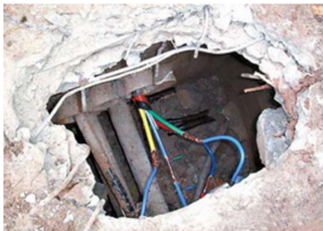
Figure 6: Cables damaged by theft
