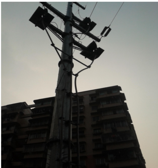
Figure 12: Shuhui Line 110 kV cable termination, pole #31 of Tongda farm produce market
