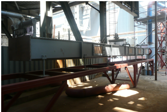
Figure 5: The 312 kW heat exchanger with the following elements visible (from left to right): cooling water manifold, pipe cleaning water manifold, inspection windows, a liquid trap, and the outlet flue gas duct
