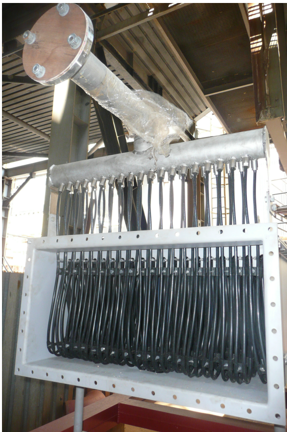
Figure 6: The interior of the heat exchanger with PFA coils and the cooling water outlet manifold
